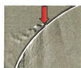
Venting of Large Tanks (identified with FLIR camera)
