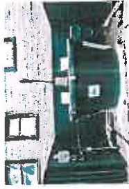
Earth Tub system behind LEED-certified Hot Italian Pizzeria and Pizzeria Bar in downtown Sacramento
