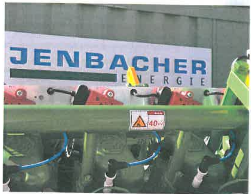
The sale of electricity generated from landfill gas by the Jenbacher engines at Catawba County's Blackburn Landfill provides the county with a reliable source of revenue from renewable energy. Source: Catawba County
